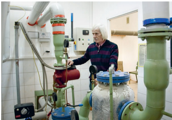
Modernised heat exchange system in a school of Częstochowa
